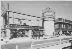
The two furnaces for Pipestills 5 & 6 rising near the north refinery road with a concrete smokestack in center that will be 350 ft. high and serve both furnaces.
